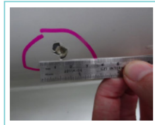
Photo 4: Chip with significant impact damage
