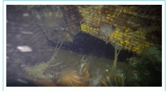
Figure 3: Intake structure broken grid due to jelly fish
