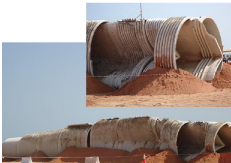
Figure 5: Collapse of an intake pipe due to buckling
