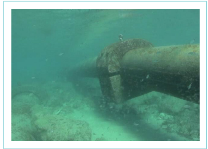
Figure 8: Outfall pipe rising towards the sea surface due to entrained air. At the left, the intake pipe can be seen. Both pipes were initially placed in the same trench, but buoyancy forces lifted the outfall.
