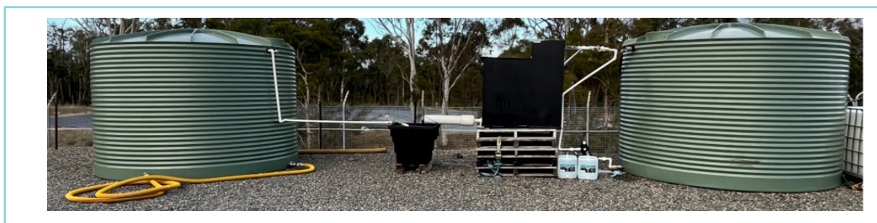
Figure 5: Photo of treatment system & associated monitoring at site for study 2
