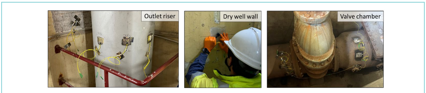
Figure 6: Photographs showing examples of sensors installed at various locations throughout PS001 (from left to right): outlet riser; dry well wall and valve chamber
